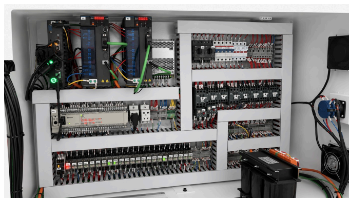
Electrical cabinet — servo drives, PLC and switchgear
